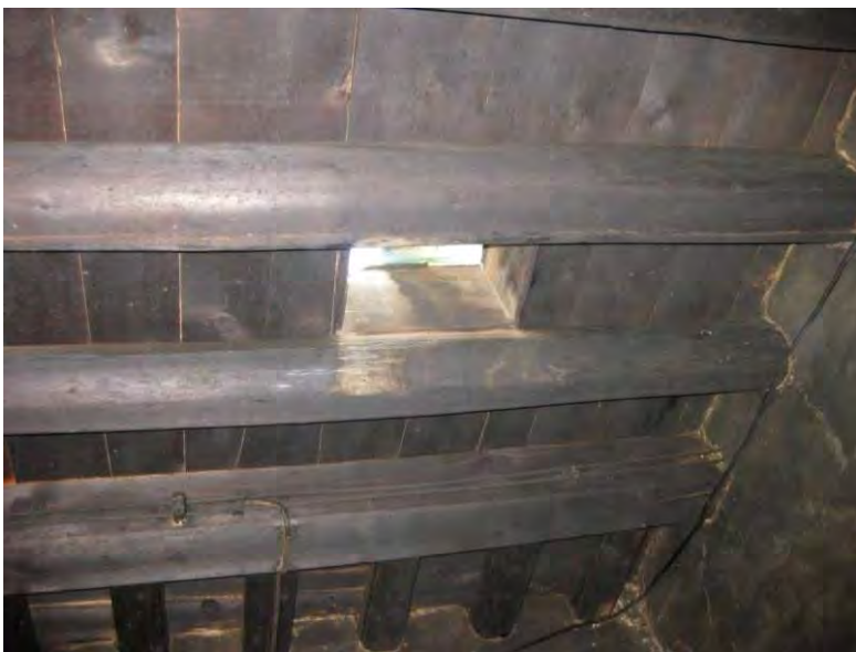
Figure Four. Kitchen ceiling and walls blackened by smoke.
