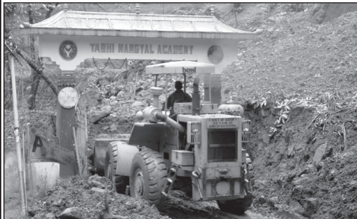
A bulldozer labours away to clear the debris which all but buried the TNA main gate yesterday and blocked the Public School's main entrance for all traffic. [turn to pg 3 for update on the slide]
