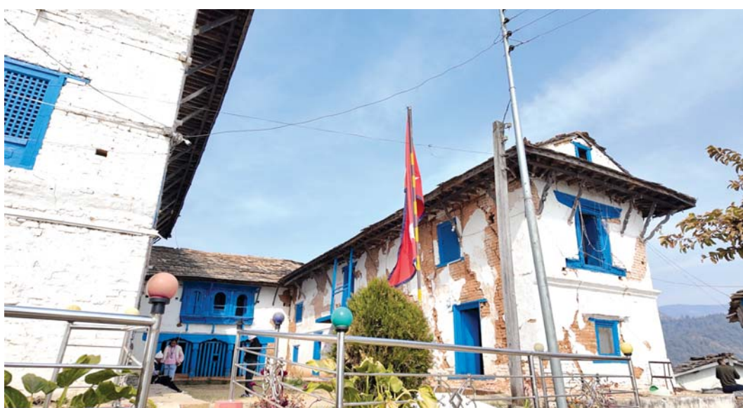
The heavily damaged police station is still flying the flag as it awaits repairs.
