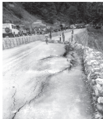
Although not looked after by the Roads Bridges Deptt., the 9th Mile slide is one example of a problem spot that evades all solutions
